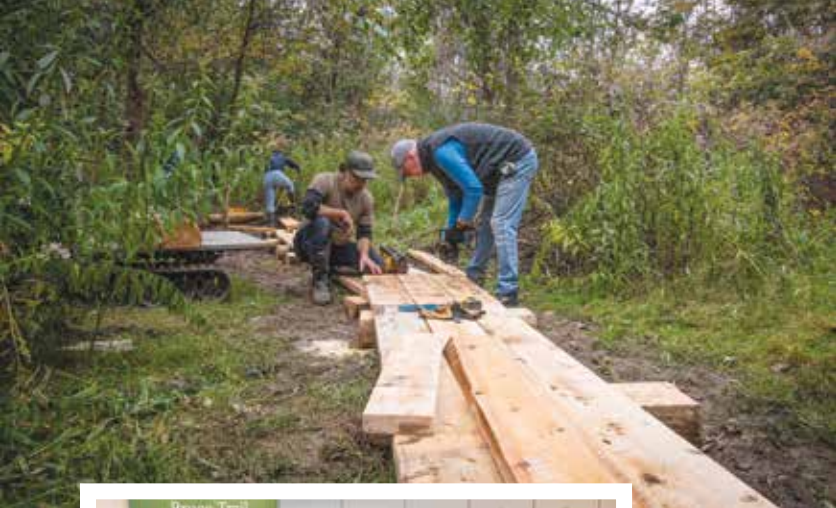
◀ In the fall of 2023 members of the Trout Hollow Trails Association finished building a long boardwalk at the west end of Meaford's Muir St. in the Bighead River Valley. Regional Tourist Organization #7 provided a grant to cover the costs of trail design and materials. PHOTO BY ROBERT BURCHER.
