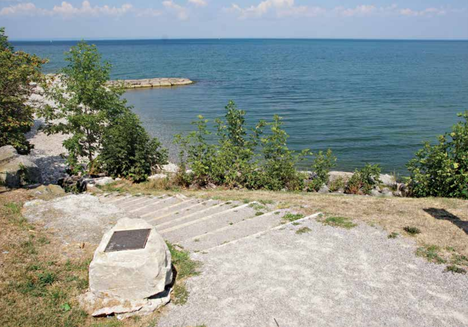
▲ Thanks to Walter Muisse, the shore of Lake Ontario is protected here by special construction features. PHOTO BY MIKE DAVIS.
