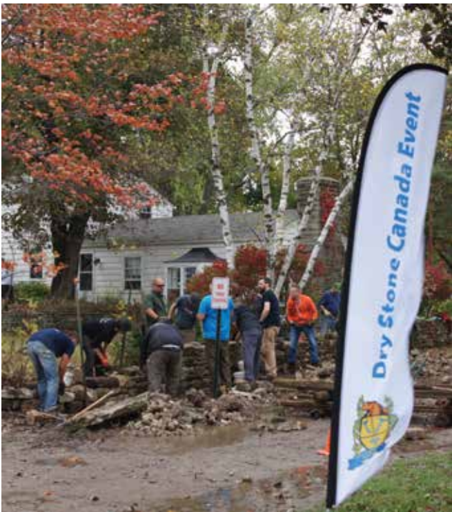
▲ Dry Stone Canada held a walling workshop on Oct. 14 to 15 at Scotsdale north of Georgetown, to repair a section of wall surrounding the Bennett house.
