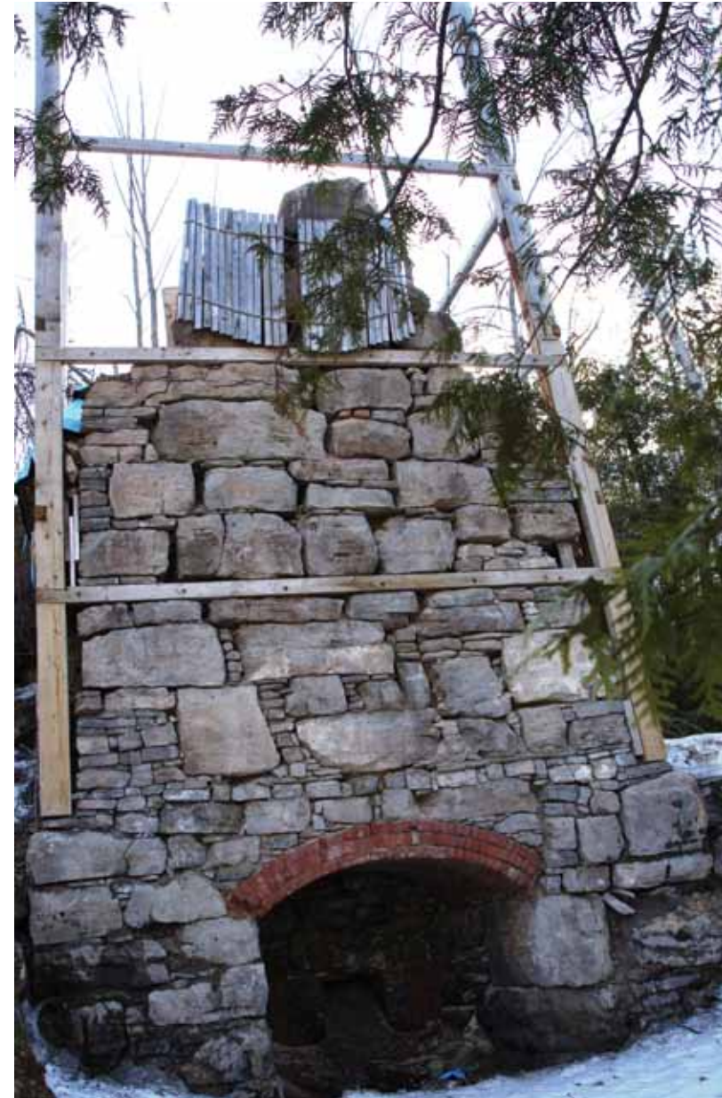
▲ The front face of the Draw Kiln after restoration and stabilization to date. The Society would like to restore the structure to the top wooden rail. PHOTO BY MIKE DAVIS.
